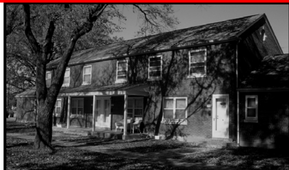
✗ The long unbroken roof and facade are monotonous. Windows and columns are incorrectly proportioned, and the entrance on the right is poorly defined.
