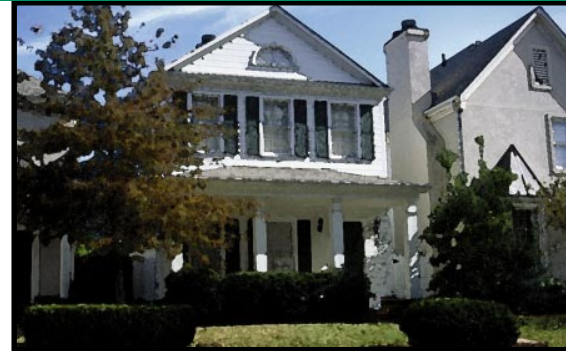
✓ The eaves, gutters and chimneys extend as much as 2'-0" into the side yard setbacks, yet remain 3'-0" minimum from the side lot line.
